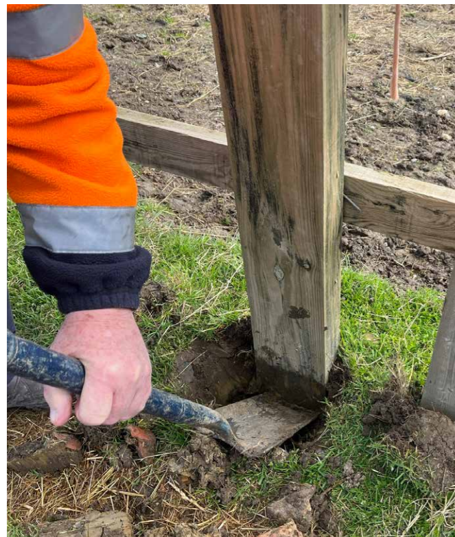
No evidence of Tanasote® treated post failure at point at ground contact.
